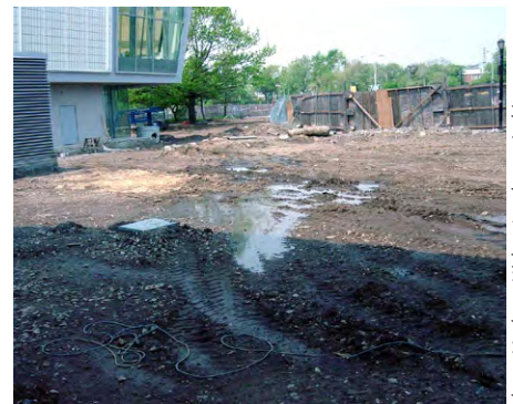
Compacted soils result in poor drainage and reduced air movement
