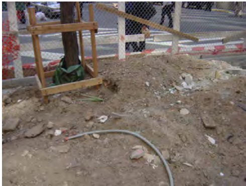
Example of inadequate tree protection
