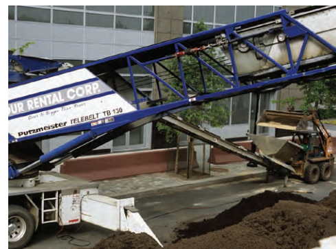
Soil Telebelt enables soil installation in elevated or inaccessible places and prevents compaction from truck tires
